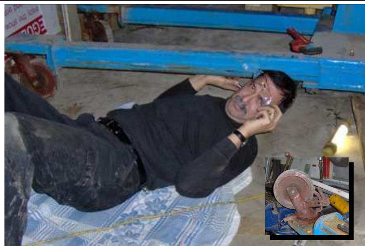
Thanks to Carl Bergsneider for repairing the broken engine hoist - one of the wheel mounts had been broken and left for repair, and Carl kindly took on that responsibility.
